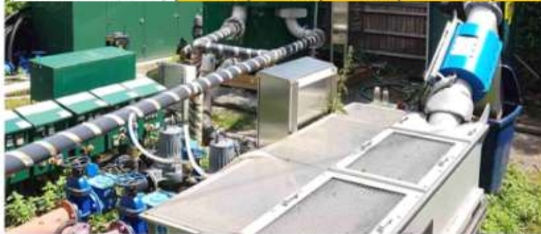
Photo of a typical groundwater treatment unit.
